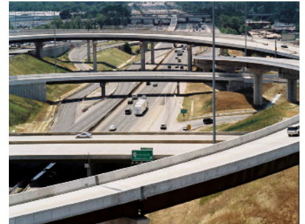
Shirley completed construction of the $110 million Phase II/III Springfield Interchange Project, designed by Dewberry.
